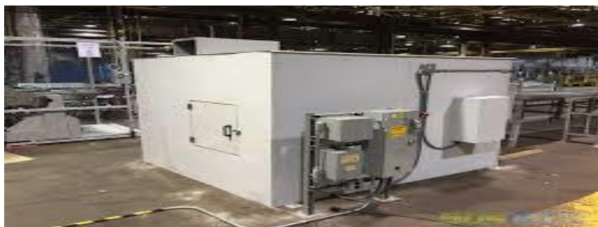
Acoustic enclosures of power plant
