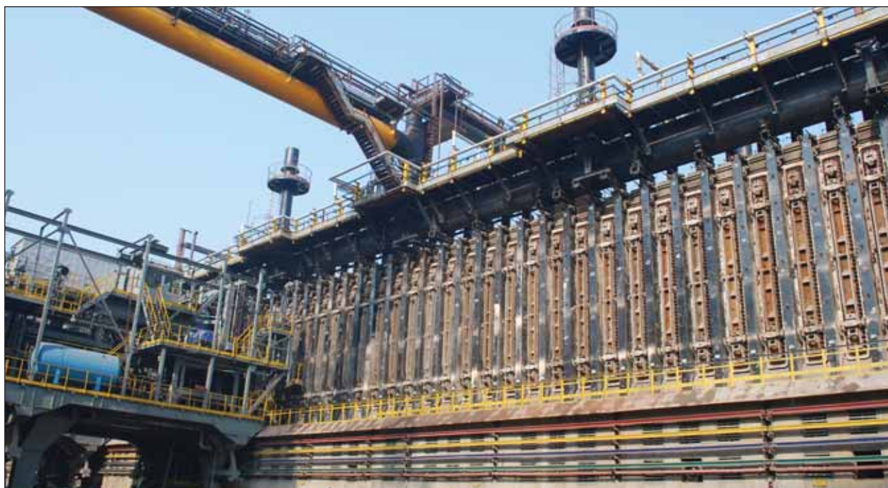
The newly built Coke Oven Battery of SAIL's IISCO Steel Plant under Modernization and Expansion Programme.
